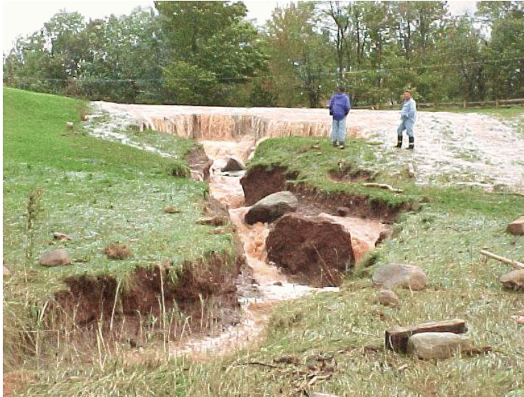
Figure IV-47: Damage to north emergency spillway on the C.D.Lane dam as the result of flows from tropical storm Floyd
