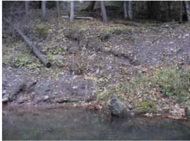
Figure 5. Eroding glacial lake clay along the stream bank and valley wall, across from the Fischzang property (see also MU17, monitoring cross-section 3).
