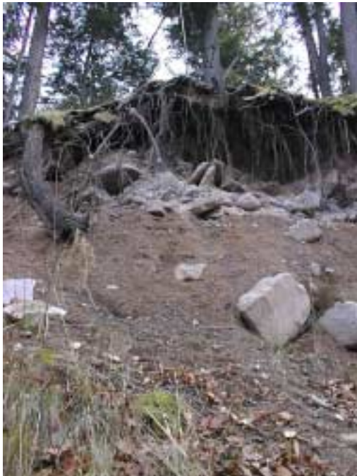
Figure 6. Eroding kame terrace (ice contact deposit) composed of silts, sands, gravels and boulders along the stream bank across from the Foss property (see also MU8, monitoring cross-sections 11, 12 and 13).
